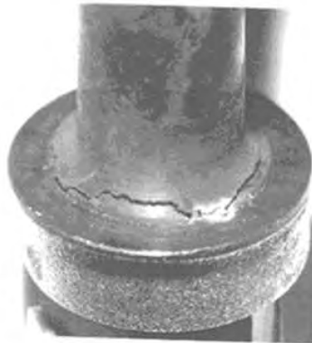
Figure 1.7: Irradiation-assisted stress corrosion cracking has resulted in cracking at the head of a baffle bolt. From [9].
