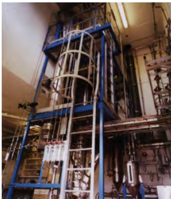
Figure 1.3: Pilot MTO plant [24]
